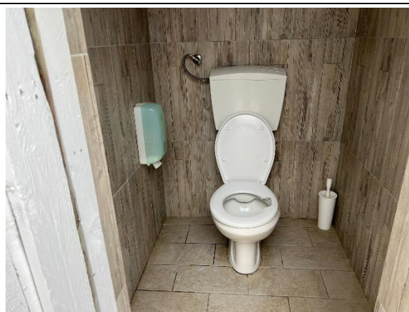
No, per door/confined space for a wheelchair resident
